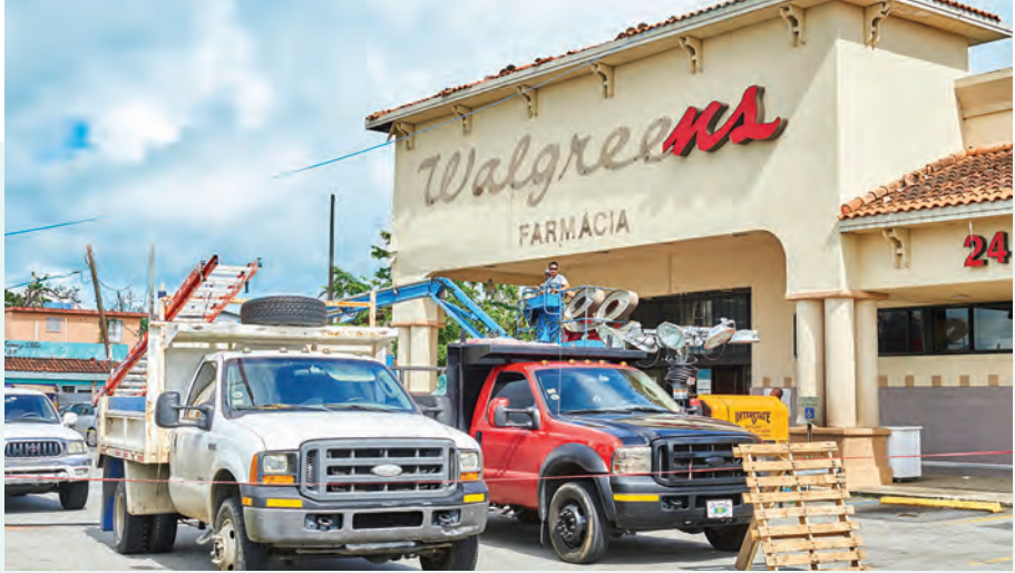
Walgreens worked to repair damage to stores in Puerto Rico following Hurricane Maria.
