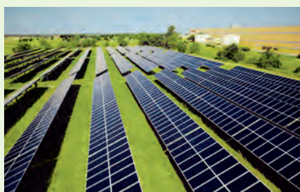
Solar panels at the Walgreens distribution center in Waxahachie, Texas.
